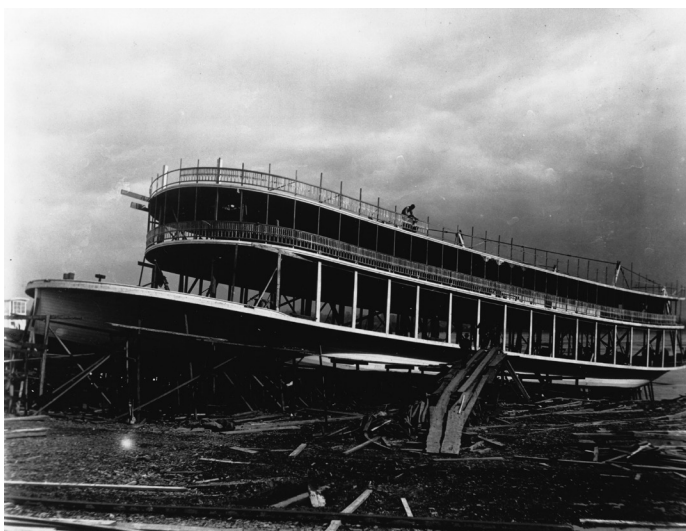
First steamer J.S. under construction at Howards in 1901. Built without staterooms but with a dance floor, she was to run as a day packet with occasional moonlite excursions. For further details, see "Deck Outline Lights and Steam Calliopes" on page 43. Hull was 175x33x5.5 Engines 16's with 6 ft. stroke.
