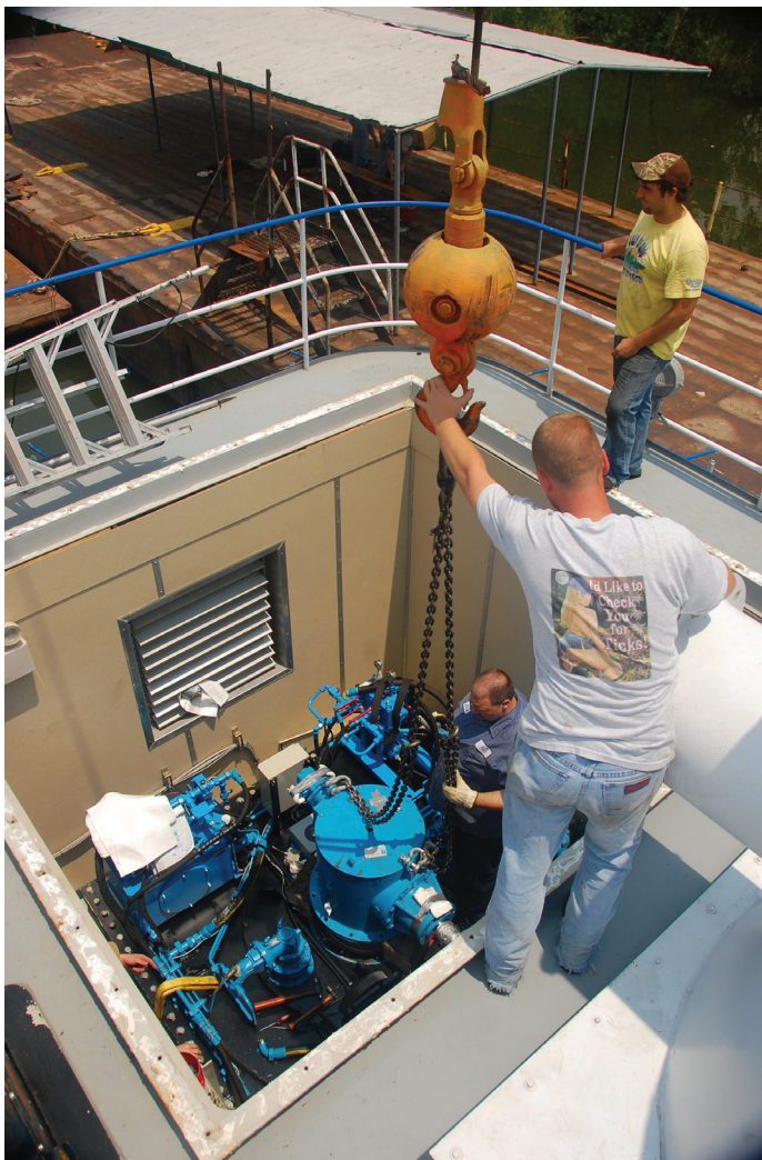
Exchanging a Z-drive propulsion unit in one of Southern Towing Company's new towboats.
