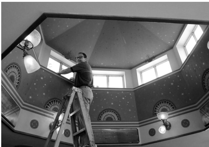
Jerry Hay cleaning the window frames after the Tiffany stained glass was removed.
