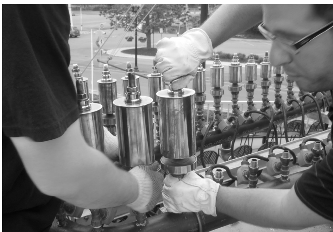
Dave Morecraft and Anthony Benedetto install copper whistles on solenoid valves. The dimensions and design of the whistles are accurate Thomas J. Nichol reproductions.
