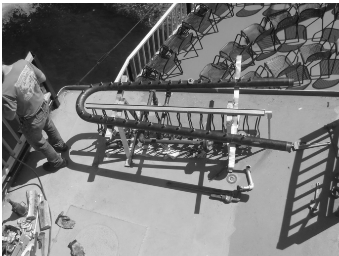
Manifold for new Morecraft calliope after its positioning on roof of MINNE-HA-HA during the week prior to Memorial Day. Solenoids and valves were placed soon afterwards.
