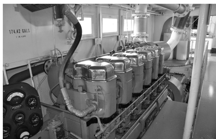
Cylinder heads of the starboard 750 hp Enterprise diesel.
