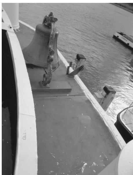
Replaced decking on forward end of boiler deck. Search lights and bell were removed and refurbished.
