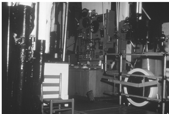
Tool room, paint locker, steam dynamo at rear of engineroom.
