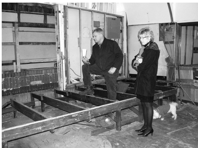
Mike Fitzgerald and Linda Harris examine progress during removal of old bandstand and restoration of original flooring.
