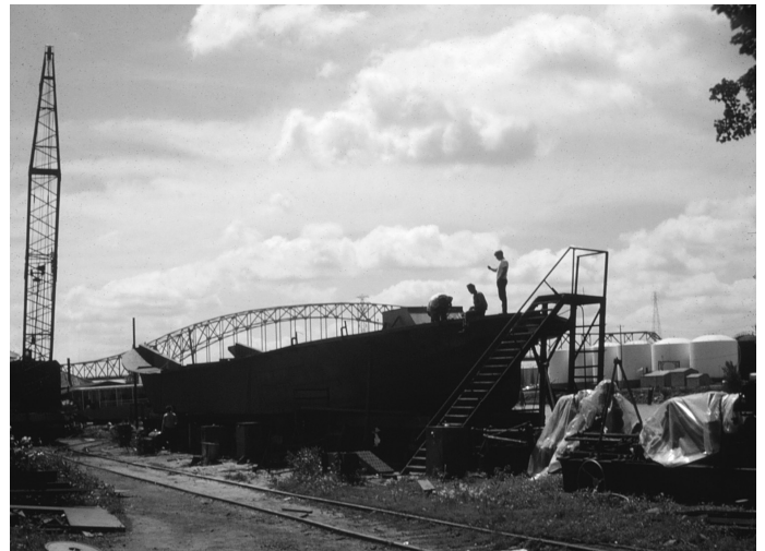
JULIA BELLE SWAIN under construction at yards of DBBCo., June 18, 1970 in Dubuque Ice Harbor. Editor's photo.
