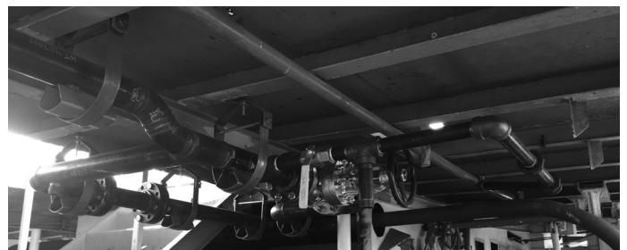
New main steam line and valves have been installed.
