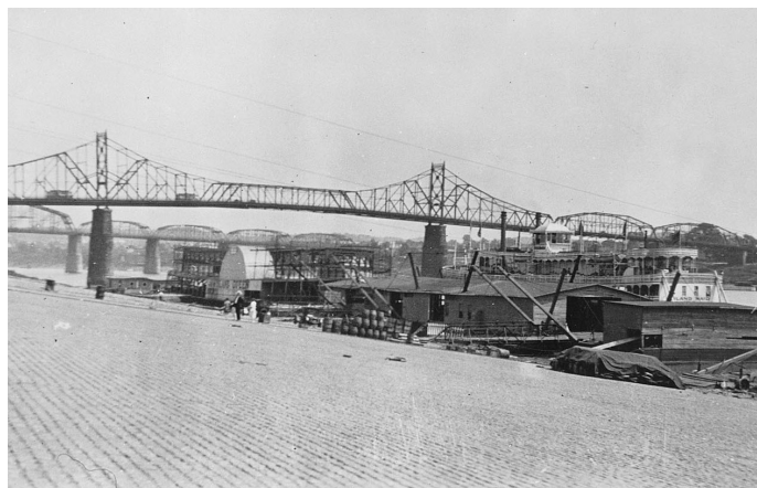
ISLAND QUEEN framed to third deck (balcony/mezzanine) level with ISLAND MAID landed below. Boilers had already been placed at Gallipolis and Barnes engines from Cincinnati were also installed. Photo by Murphy Library, UW-LaCrosse.
