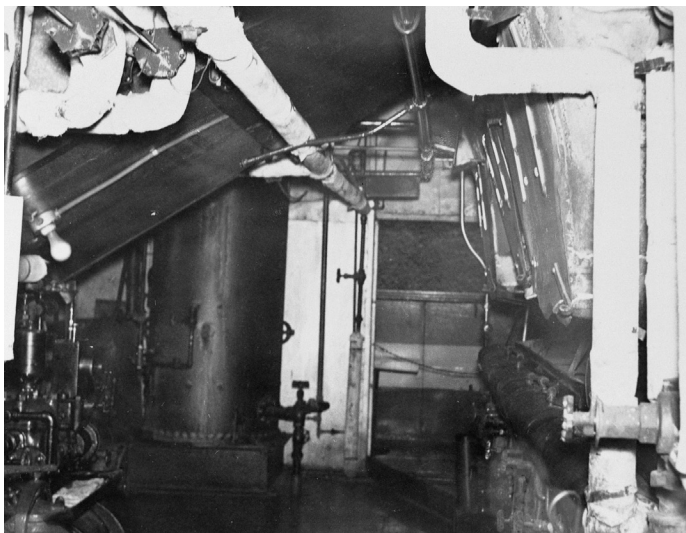
AVALON’s fire box or boiler room. At the time of this story, she was oil-fired, and the fireman always kept a watchful eye to make sure “she didn’t smoke too much.” Preacher was adept at firing with coal, starting on the river at age 14. He fired on the CAPITOL when she came out in 1920, and on IDLEWILD in her pre-AVALON days. Murphy Library photo.
